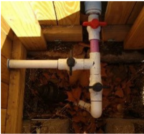
Figure 27. Cistern pipes were damaged by freezing temperatures
