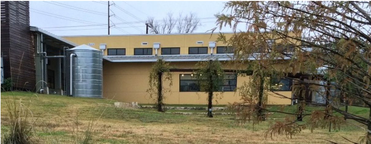
Photos showing installed tanks in reference to building and each other.
