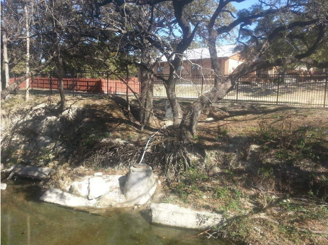
Erosion Inspection Site – 400 W. Live Oak Street
