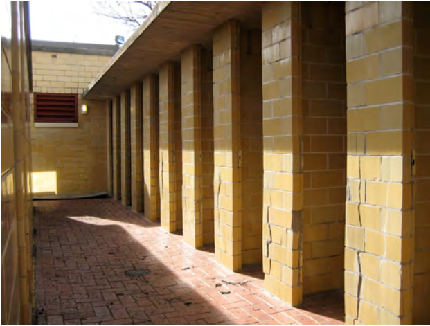
Aside from the masonry deterioration, some of the Women's Dressing area seems cramped and dank. Regular swimmers report that this area is rarely used.
