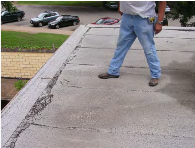
Blistering of roof membrane noted in several areas.
