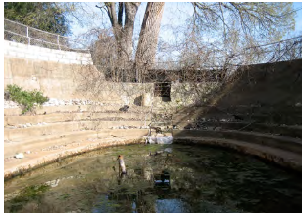
View towards Pool. Stonework should be removed to reopen slot in amphitheater, allowing flow into recreated spring run.
