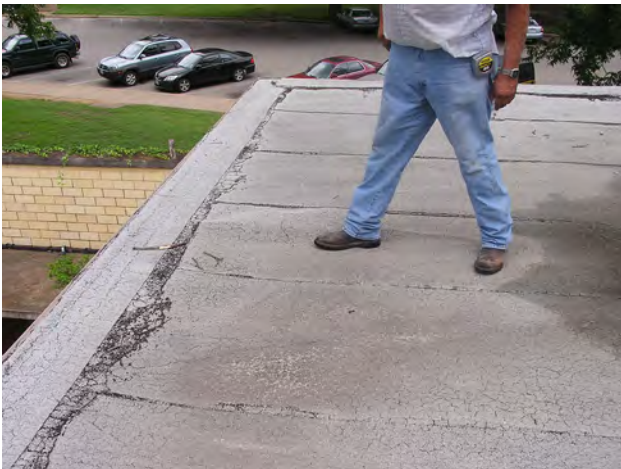
Many of the subordinate roofs are flat, and are surrounded by parapet walls. Because they are designed with a primary roof drain and no overflow drain, they do not meet today's code (above). Some of the roof membranes are pulling away from their substrates and puckering (below).
