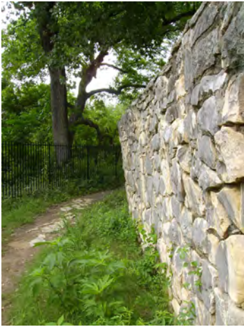
Some walls are leaning precipitously. Strategy for stabilization should account for historic preservation, long-term service and public safety.
