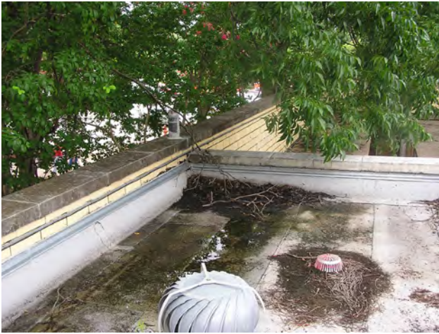
Certain roof areas are bordered by parapet walls that vary in height from a few inches to over three feet. These areas are drained by roof drains, but do not include overflow drainage provision.
