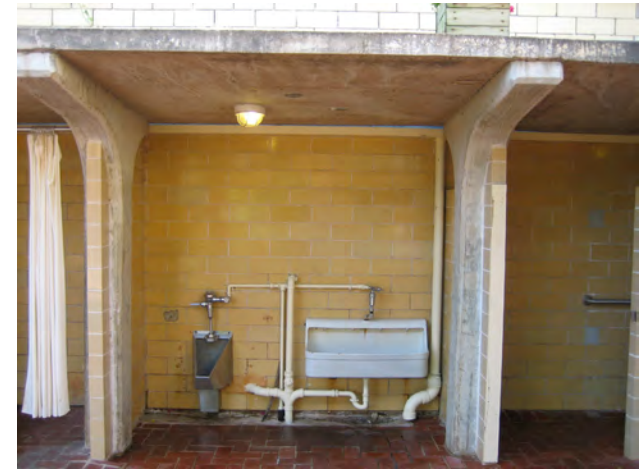
Plumbing fixtures vary in age and condition. Trough urinals (right) do not meet current code. None of the fixtures are low water-use fixtures.
