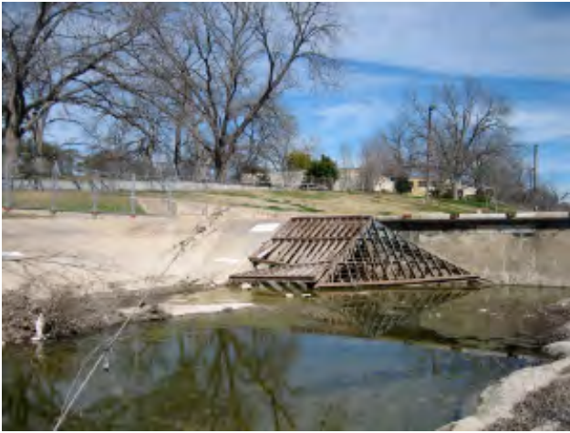
Existing inlet grate is damaged and clogs too easily.
