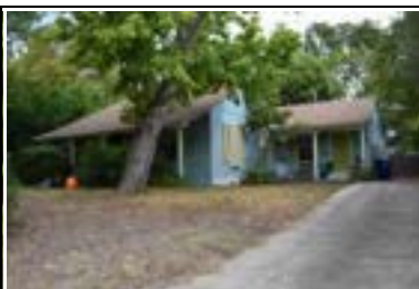
Address: 1706 W 34 St Year Built: 1950 HHM ID: 95861 NR Recommendation: Update previous district listing
