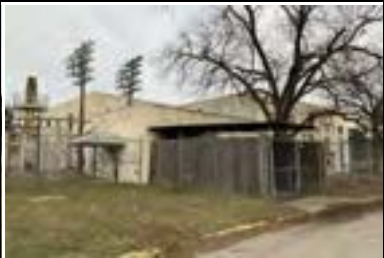
Address: 4110 Guadalupe St (C) Year Built: 1899 HHM ID: 113385 NR Recommendation: Within district
