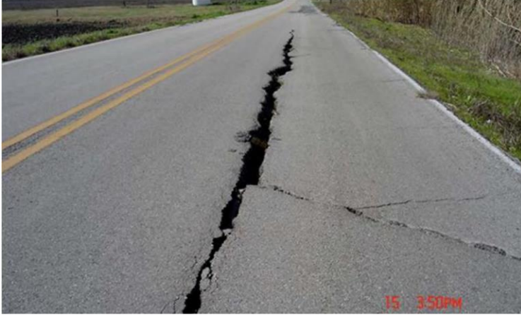
Photo of a severe pavement crack on Hamann Lane in Travis County in 2005. Photo credit: City of Austin.
